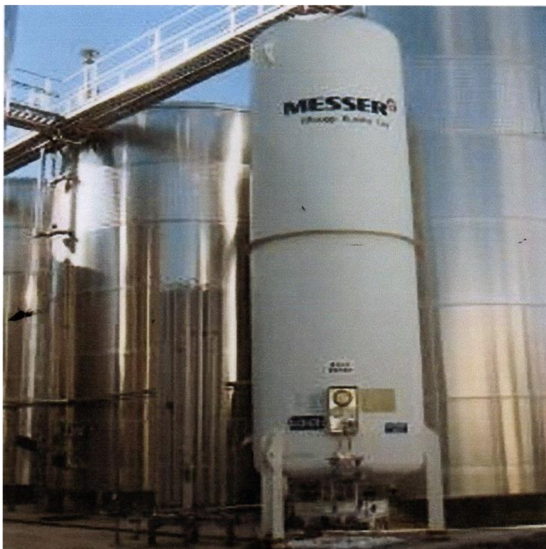
Figure 5.19 Industrial liquid hydrogen storage tanks
