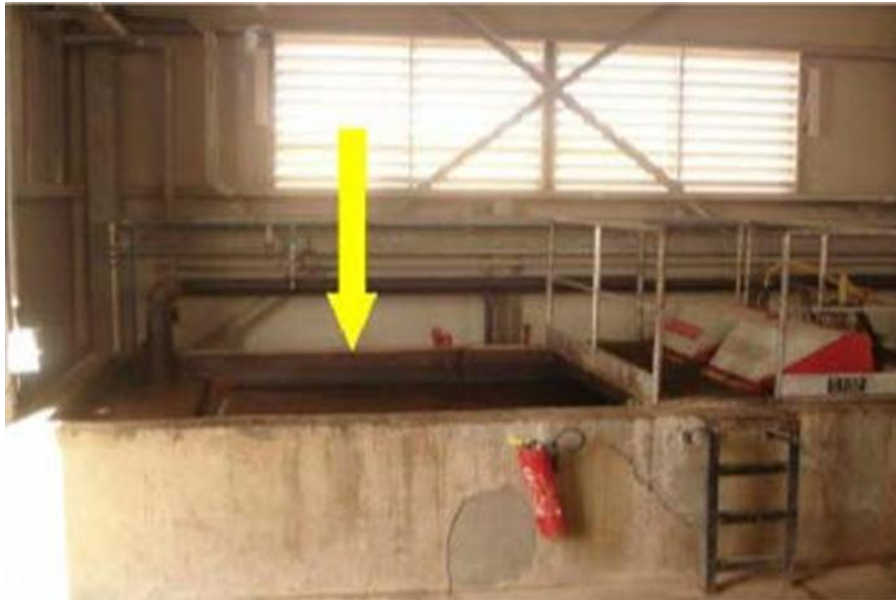
Figure 12: La cuve CPI
