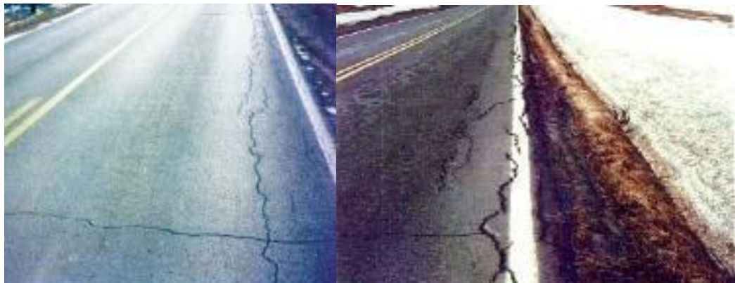
Figure 2.5 : Fissures de rives
