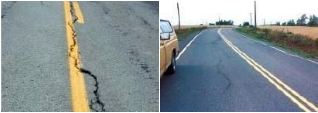
Figure 2.6: Fissures de gel
