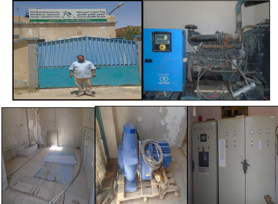
Photo II-12: Station de relevage
