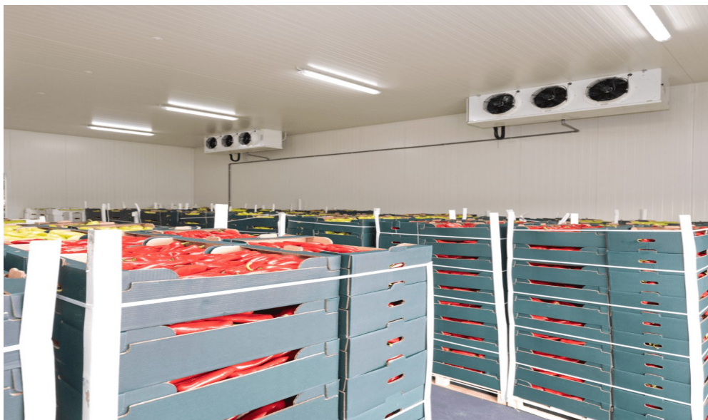
Figure III. 3: cold room storage
