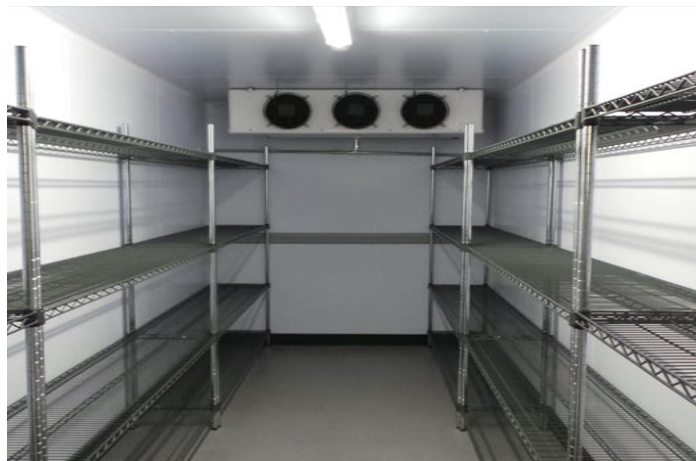
Figure III. 2: cold room from inside
