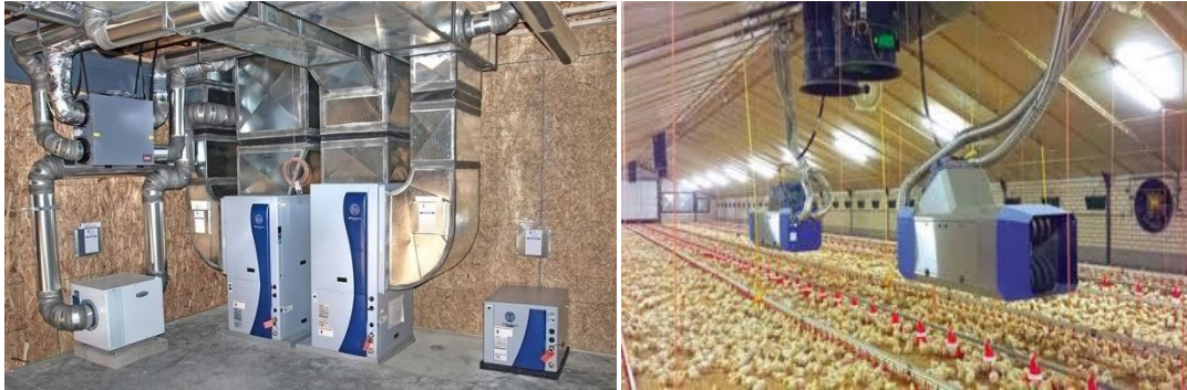
Figure II.13: Heating distribution system in poultry house.[52]
