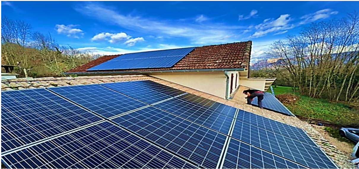
Figure (I.8): Standalone rooftop photovoltaic system supplying electricity to a remote mountainous home isolated from the national grid.
