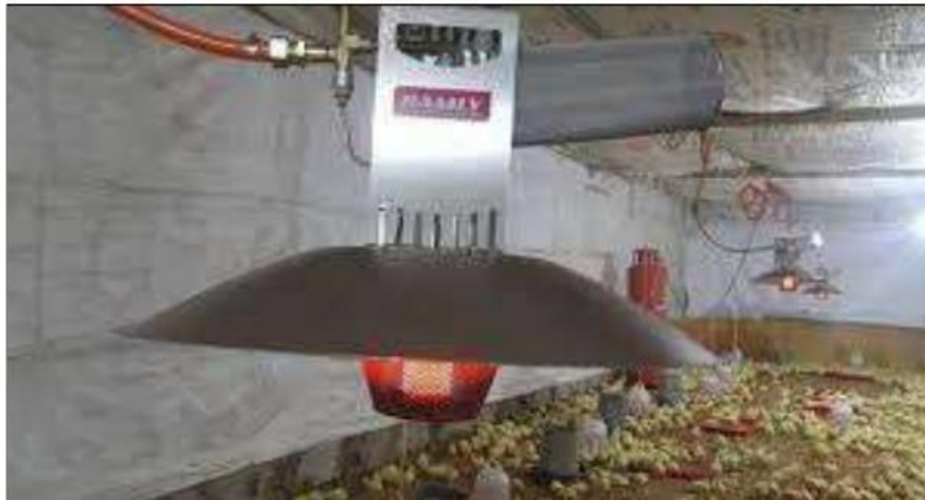
Fig II.9: Gas heaters in poultry houses [40].
