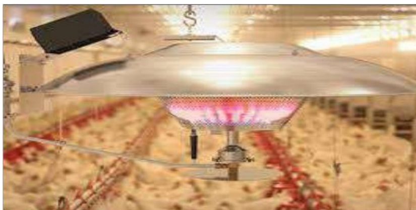
Fig II. 8: Gas heaters in poultry houses [40].
