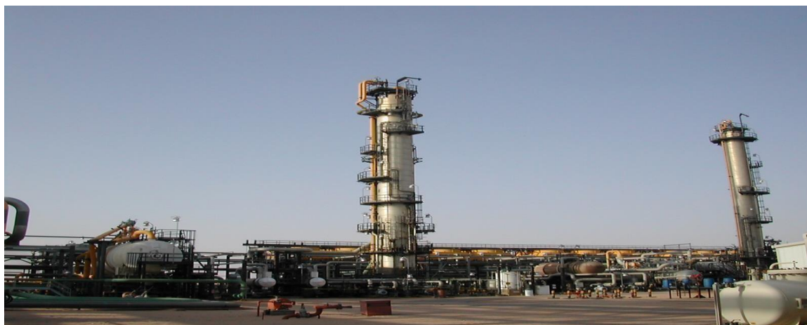
Figure II.13: La Section stabilisation basse pression.
