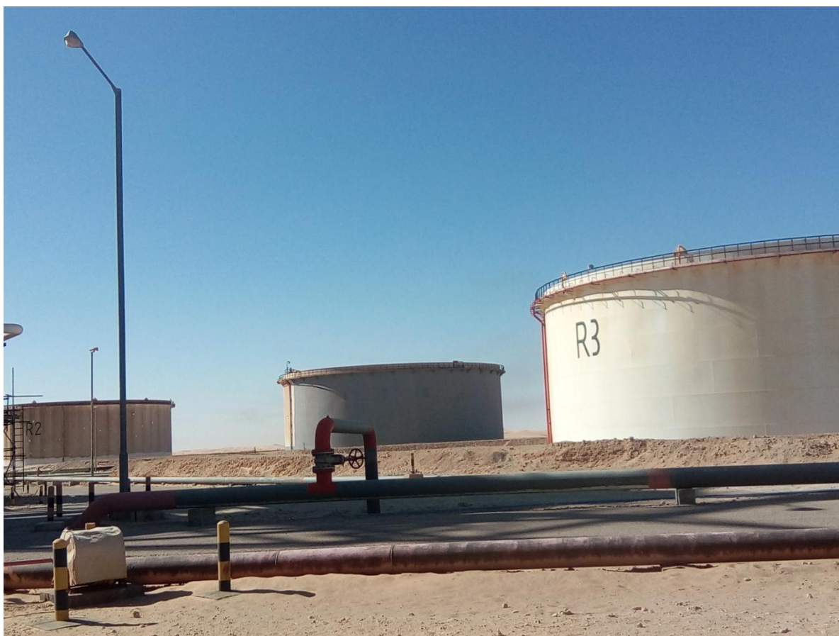
Figure II.8: Bacs de stockage .
