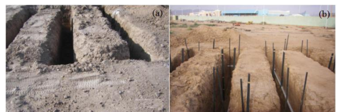
Fig.1. Experimental EAHE setup: (a) hole with a serpentine shape; (b) buried horizontal PVC pipe with thermocouples (4).
