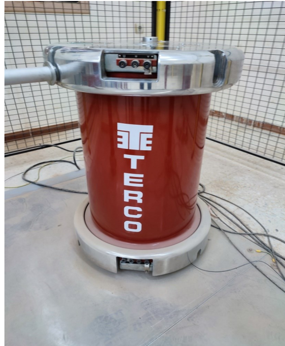
Figure 4.3: High voltage transformer
