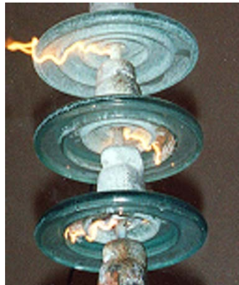
Fig. 3.34: Polluted Glass Cap and Pin Insulator string with dry bands
