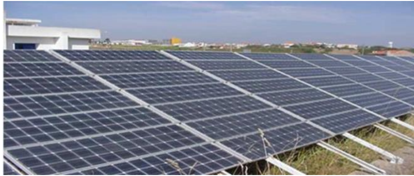
Figure I.13: Système photovoltaïque fixe
