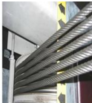
Figure I.14: Câbles de traction.
