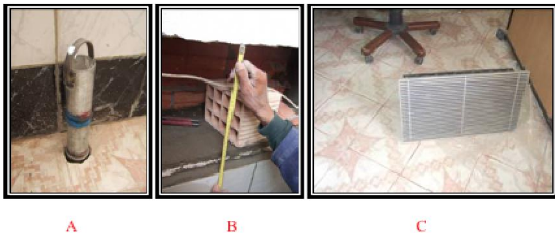
Fig.4. Realization of the over flow A, 30 cm opening to the office B Grid C
