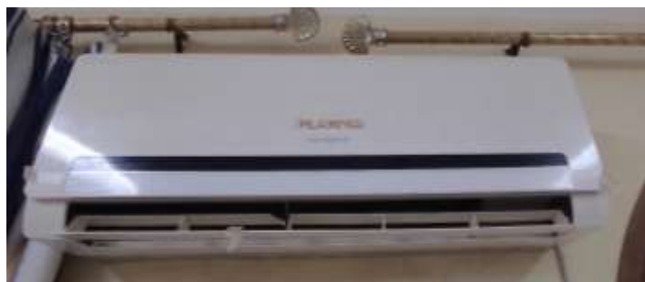
Fig (II. 8): Air conditioner AC.
