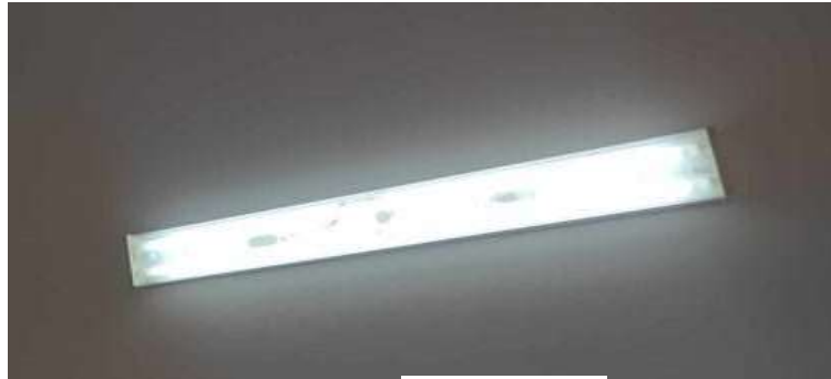
Fig (II. 9): Interior Lights
