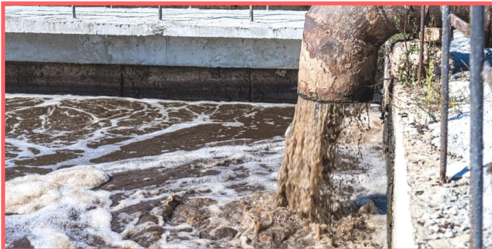
Photo02: Eaux usées industrielles [7.2]
