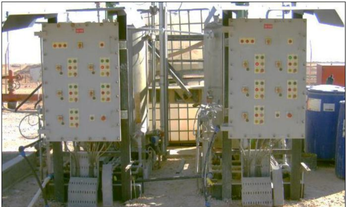
Figure III. 14: Instruments et skids d'injection coagulant/floculant.
