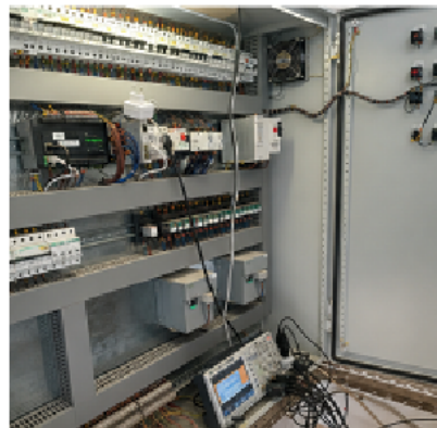
Figure 4.10: Owon XDS3204AE oscilloscope in operation at the University Hub Pumping Station, displaying the three-phase voltage and current waveforms during steady-state pump operation, March 2026.
