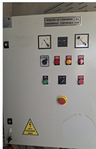
Figure 4.4: Front face of the existing starter control panel ( Armoire de Commande ), University Hub Pumping Station. The nameplate reads “Démarrage Statique 63 KW”; note that the installed motor is rated 75 kW — the panel label reflects the original design rating prior to the motor upgrade and does not affect the electrical measurements or analysis presented in this chapter.
