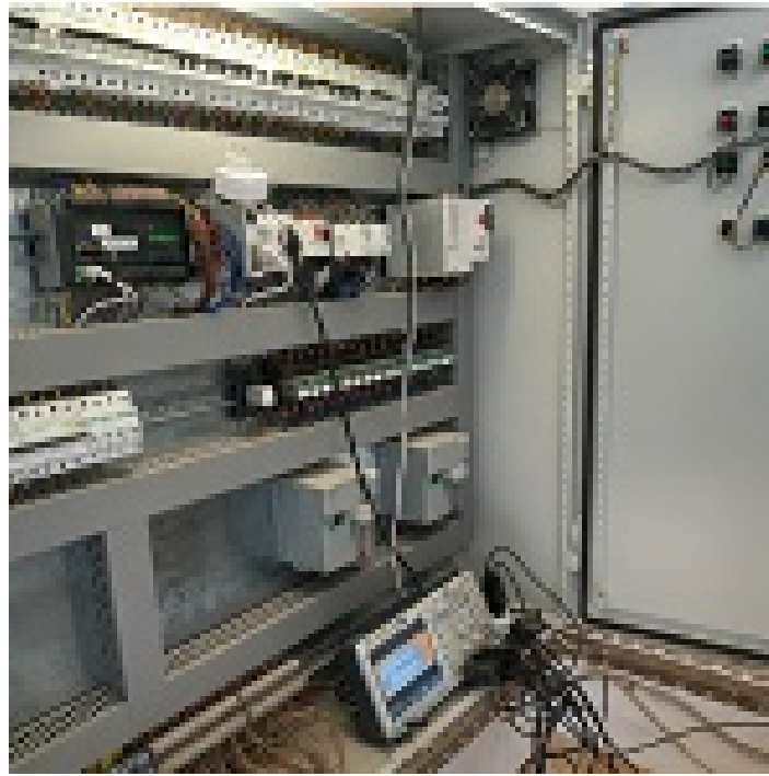
Figure 4.6: Main electrical distribution and control cabinet at the University Hub Pumping Station. The Owon XDS3204AE oscilloscope (bottom shelf) is positioned at the cabinet to acquire three-phase waveform data during the field measurement campaign, March 2026.
