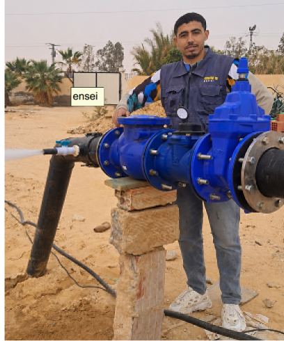
Figure 4.3: Wellhead surface discharge pipework — blue flanged riser column fitted with an isolation valve, non-return (check) valve, and inline pressure gauge, University Hub Pumping Station, El Oued.
