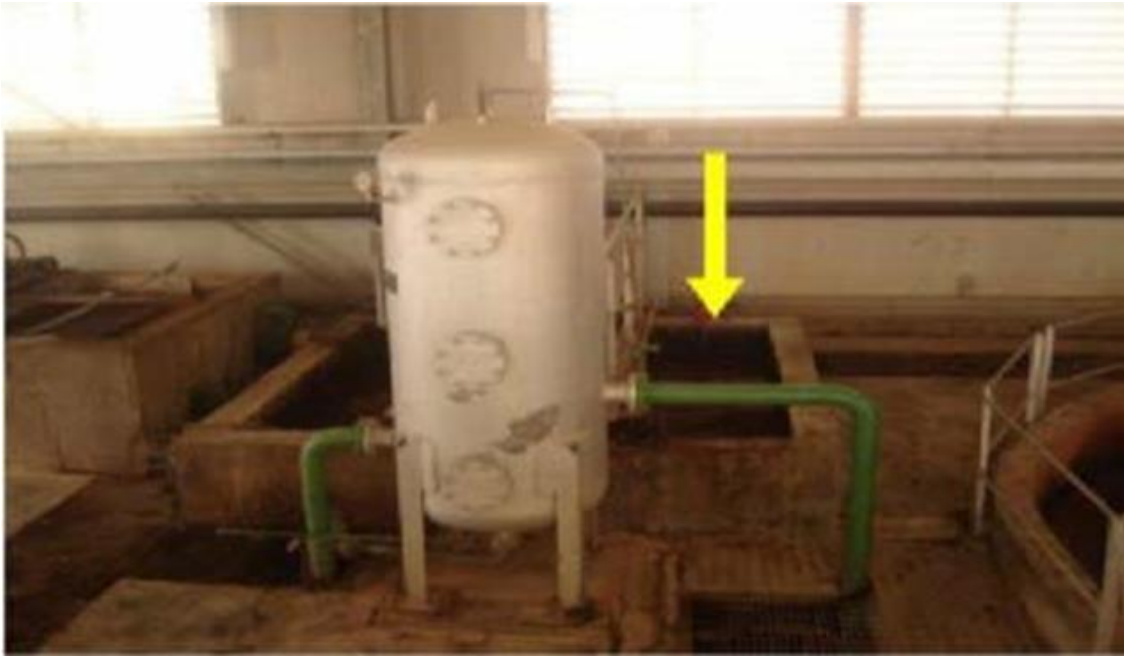
Figure I.8: Cuve de flottation
