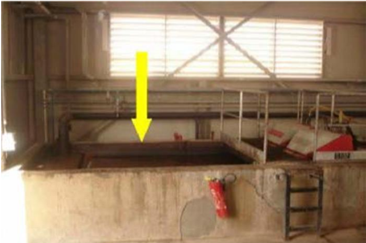
Figure I.7: La cuve CPI
