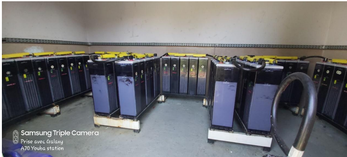
Figure II-14: Les batteries POWERBLOCS.
