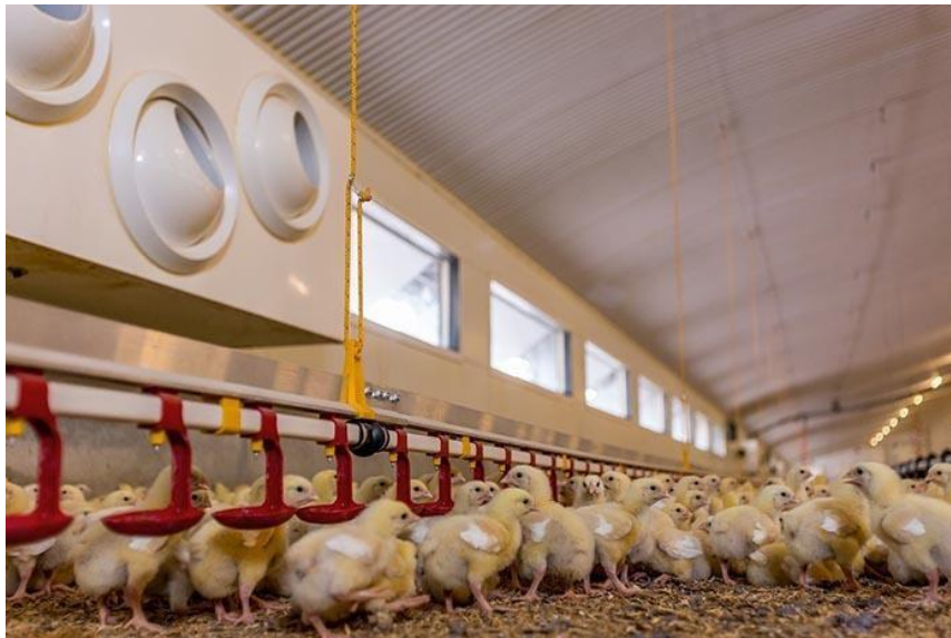
Figure I. 5: Air installation in poultry houses.
