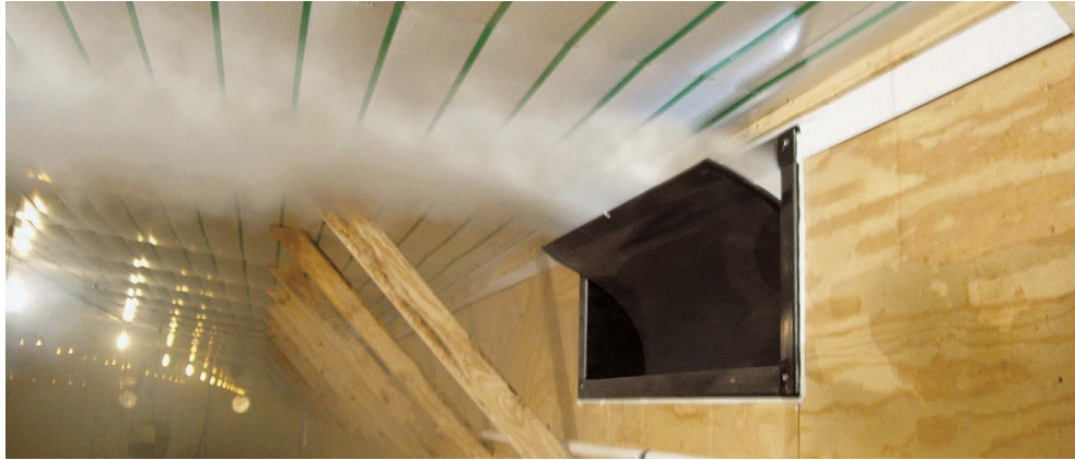
Figure I. 9: Poultry sidewall inlets - wall vent poultry house ventilation.
