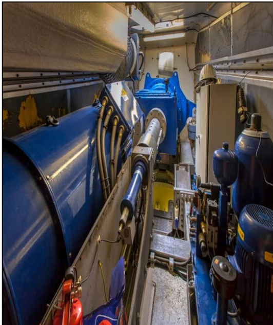
Figure I. 6: Inside mechanical components of the nacelle
