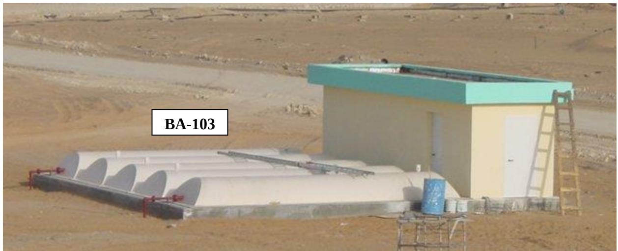
Figure III-4: cuve de relevage
