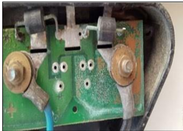
Figure 2. 21. Bypass diode fault.
