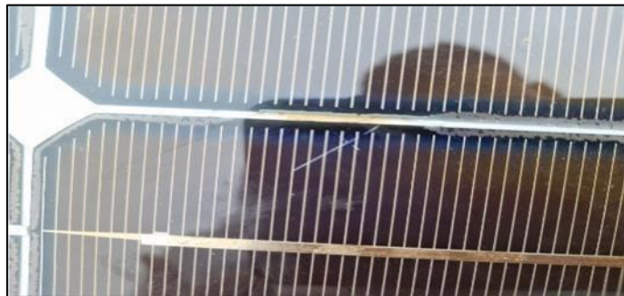
Figure 2.14. Delamination on the cell surface
