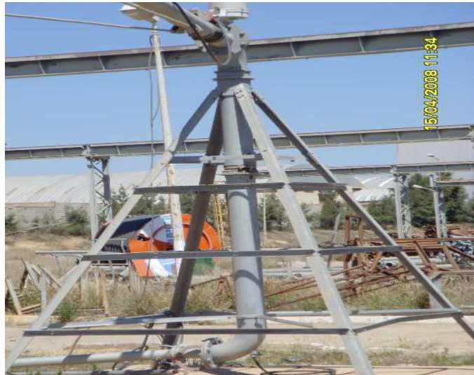
Fig.I.5: Unité centrale. Photo IRRAGRIS
