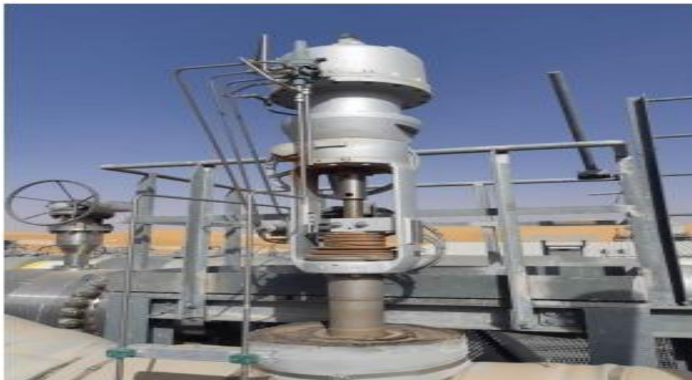
Figure III.10: Joule Thomson valve used in SH-FCP[36]
