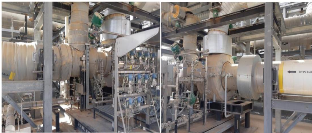
Figure III.1: The Atlas Copco MAFI-TRENCH turbo-expander/compressor assembly[29]
