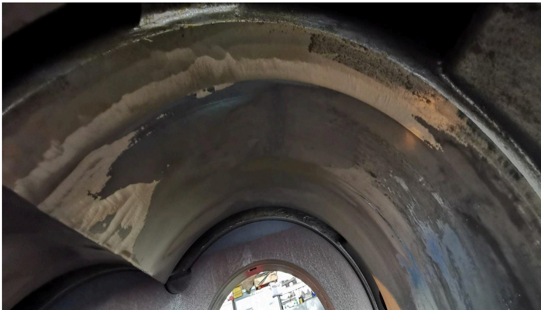
Figure II. 17: DE (Drive End Bearing) (Driven shaft side) top view.
