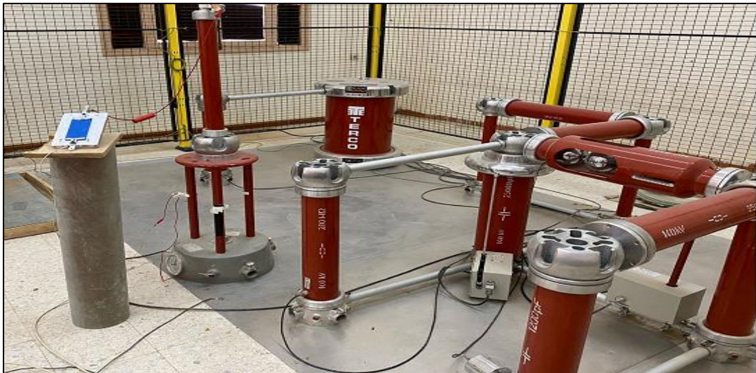
Figure III. 4. Photo of the Industrial Frequency Test Circuit.
