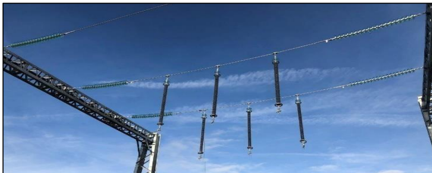
Figure II.17. Tested 400 kV insulators at Deeside station (National Grid, Deeside Centre for Innovation).
