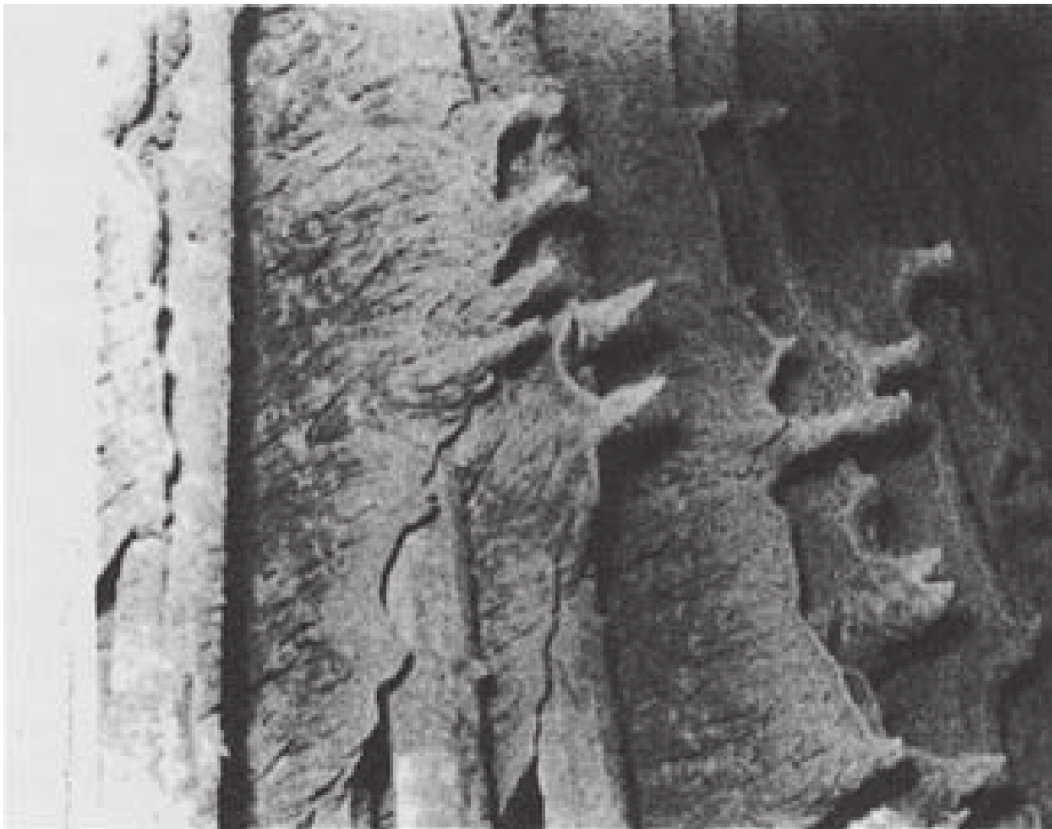
Figure 6.3: Precipitation fouling of ash particles on superheater tubes.
