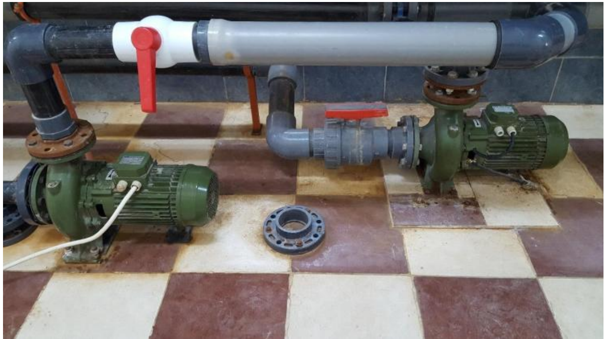
Photo III.7 : Raccordement des pompes.
