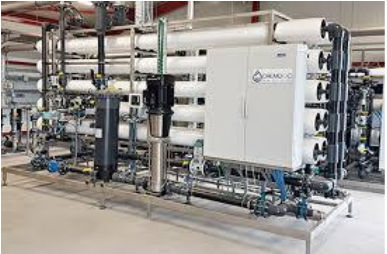
Figure I.3: Station d'osmose inverse [2]
