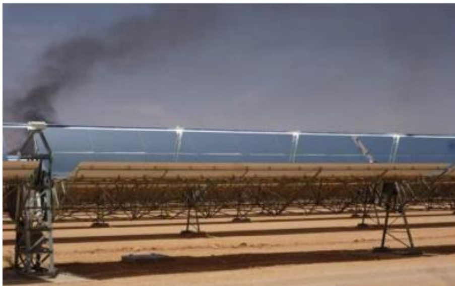
Figure I.6: Solar Field Of HassiR'Mel Hybrid Power Plant.
