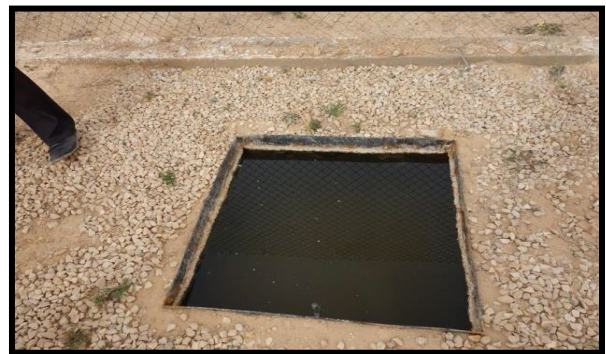
Figure II.2: Le bac Colorado
