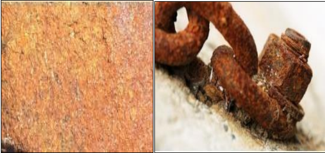
Figure III 1: Exemples de corrosion uniforme.
