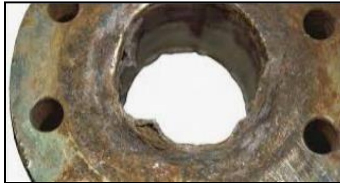
Figure III.12: Photo de la corrosion caverneuse
