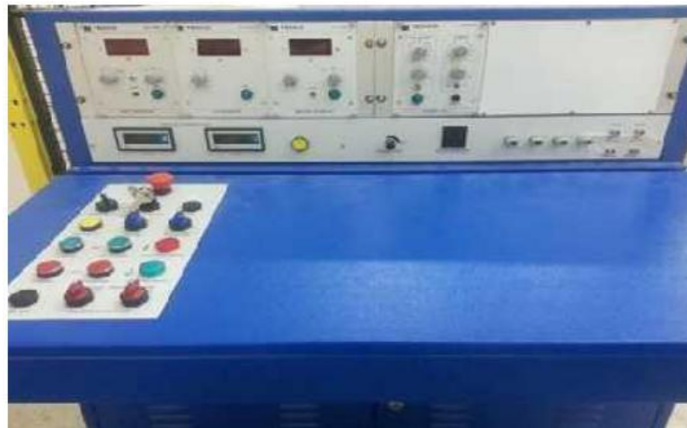
Figure III.1 — High voltage control panel used for breakdown voltage testing
