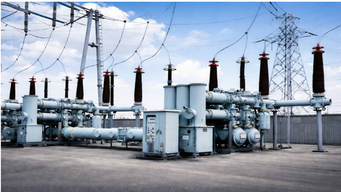
Figure I.2 A power transformer in an electrical substation [5].
