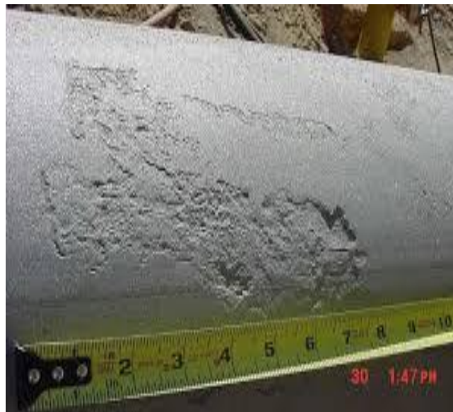
Figure 1.7: Metal affected by selective corrosion.
