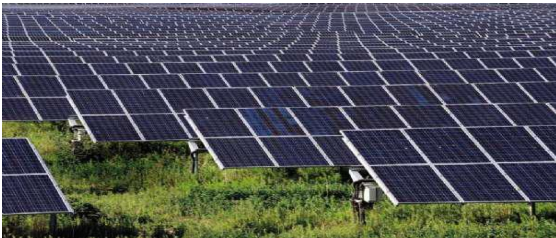
Figure (I.10): Champ photovoltaïque
