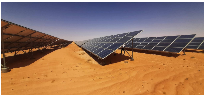
Figure 3.9: Some solar panels from Photovoltaic power center (SKTM)
