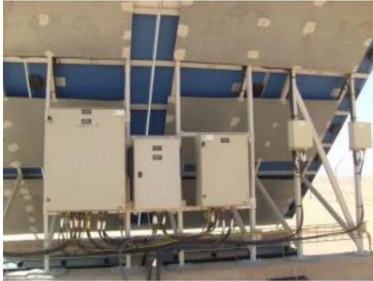
Figure II.11: Coffret de distribution
