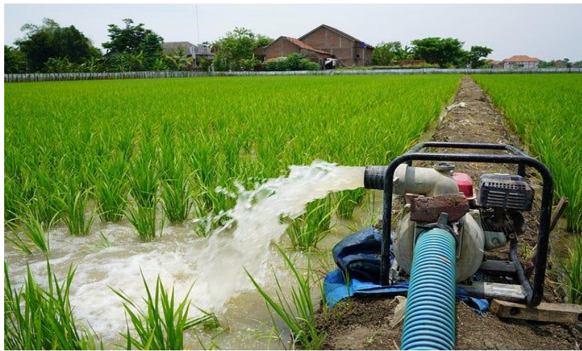
Fig II.6: Water pumping system in agricultural field
