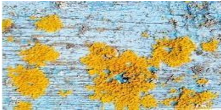
Figure 6 : Photo de la bio corrosion. [09]
