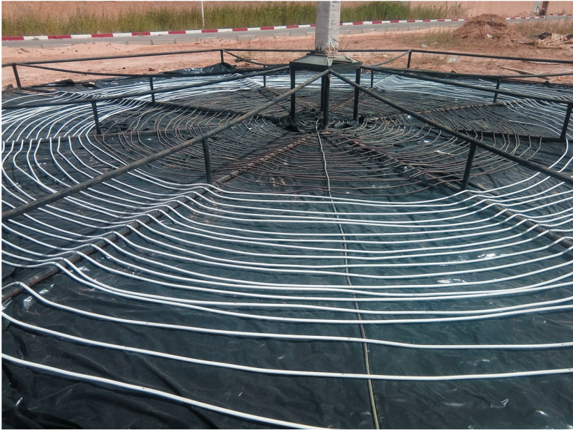
Figure 5. Picture showing the spiral thermal exchanger.
