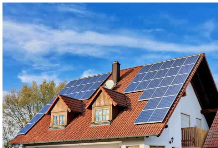
Figure (I.12): Photo of a solar panel system installed on the roof of a house.
