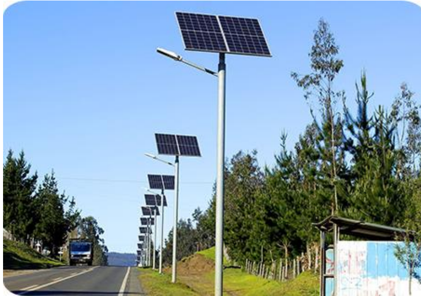
Figure (I.13): Solar-powered light pole.
