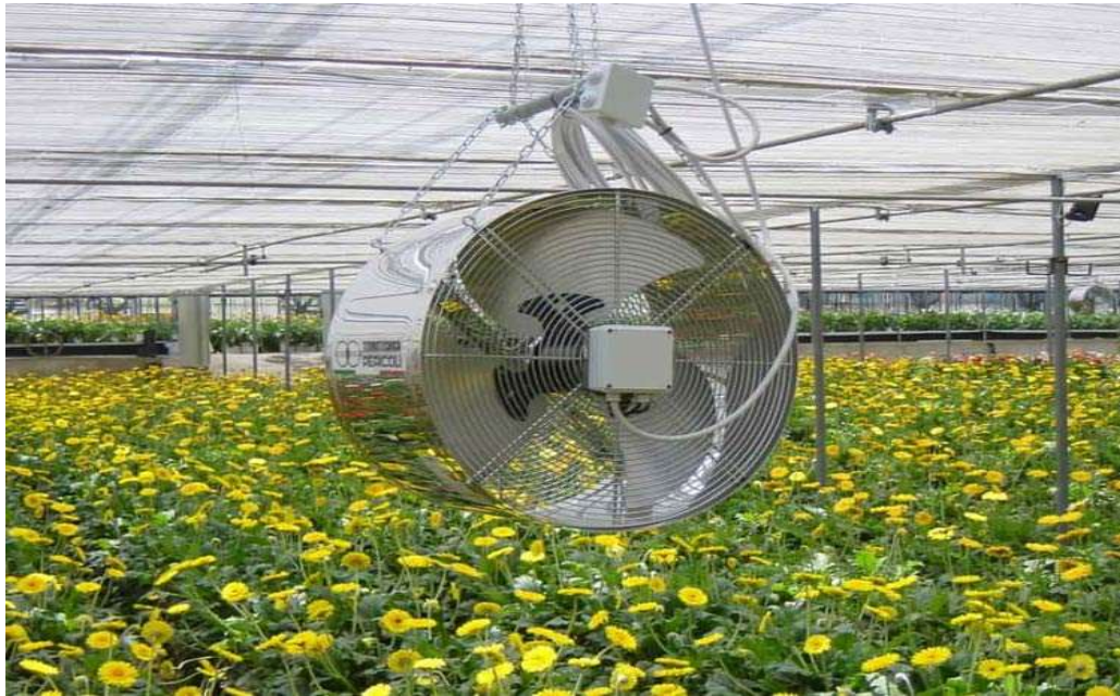
Figure I. 11: Air circulation fan [17].
