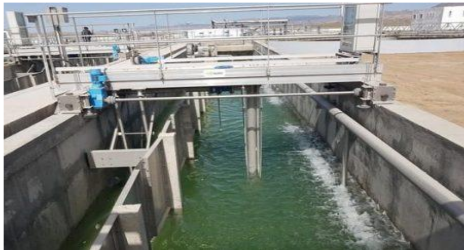
Figure 5: Wastewater treatment and purification plant - Filfila Municipality - Skikda Province .
