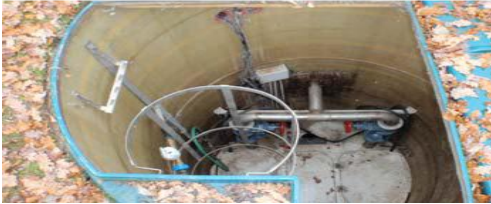
Figure 2. 5: Station de pompage [7]
