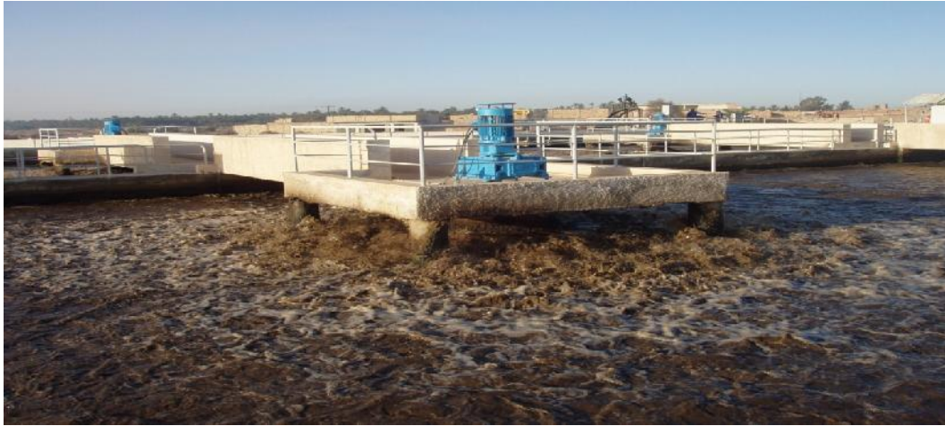
Figure 2. 6 : Station d'épuration de Touggourt [11]
