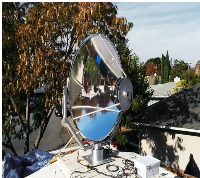
Figure 6 : Solar water heater[32]
