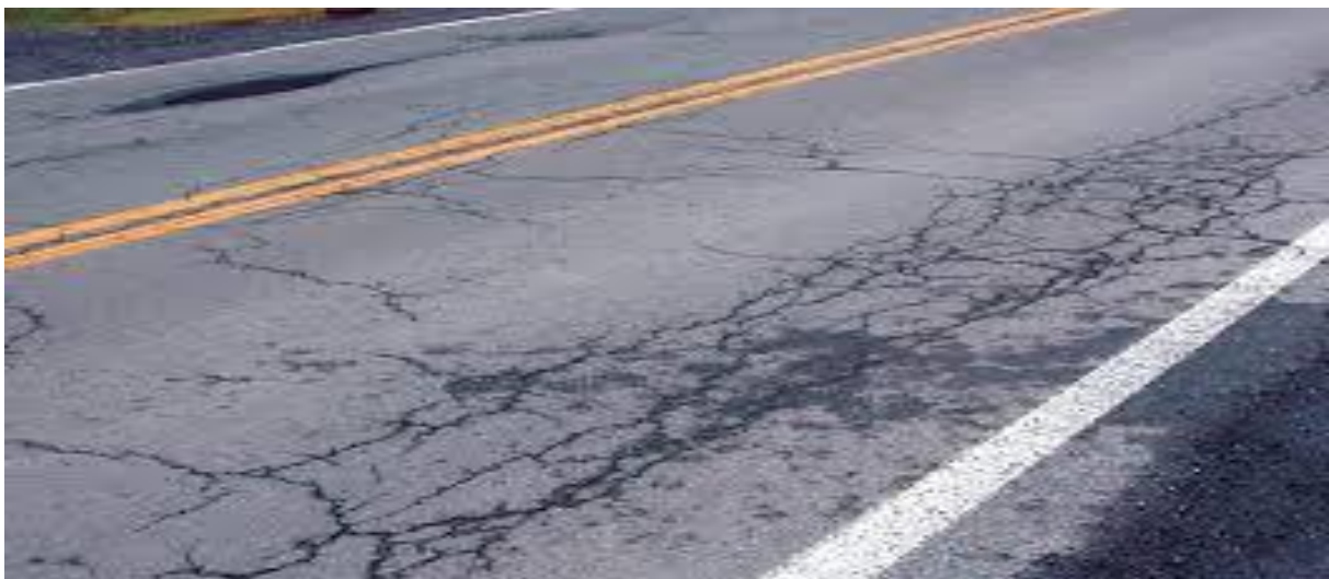
Figure 2.4: Fissures de gel
